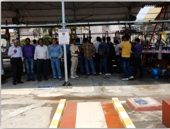
A view of pipeline operations
